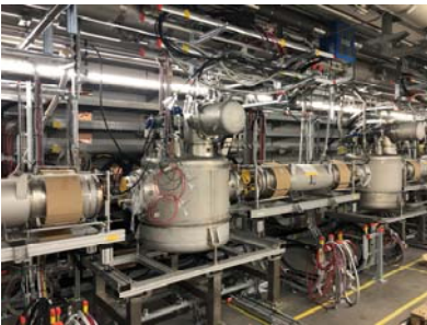
(6) Connection to cryogenic distribution system
