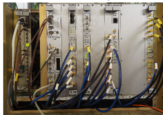
Figure 1: VME crate housing the LLRF modules for one power amplifier and its cavity.
